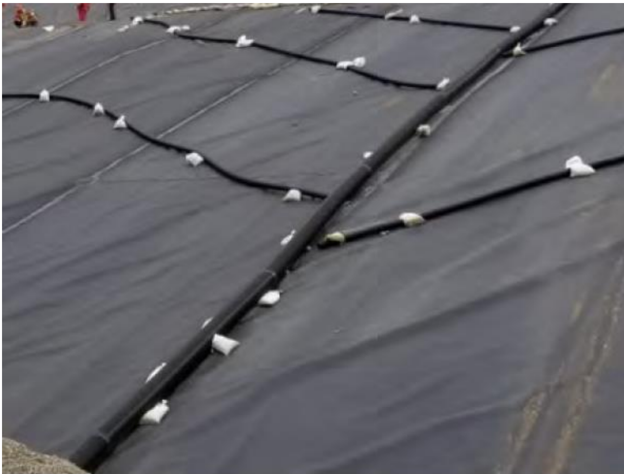
Figure 10: Lateral drainage pipes butted but not connected to drainage headers at the Eagle Gold HLF (reproduced from Smith and Konrad 2025 with permission)
